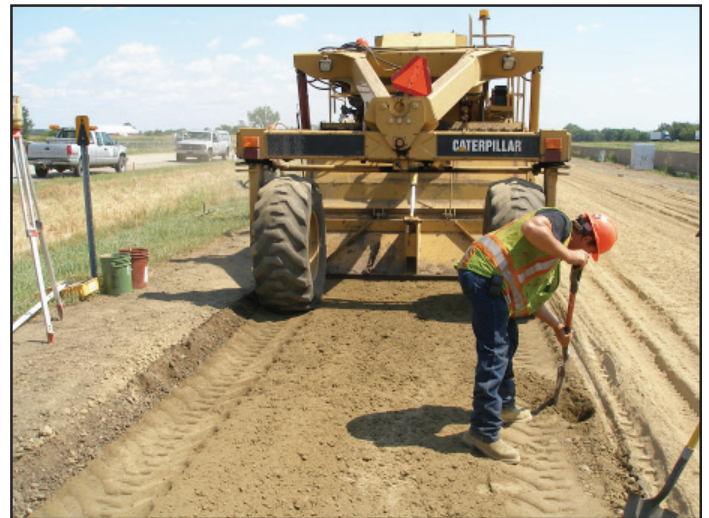
Fly Ash Stabilization: before mixing with RPM (right of Caterpillar) and after mixing (Behind the Caterpillar)
