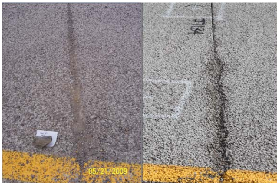
Figure 65. High severity level joint deterioration
