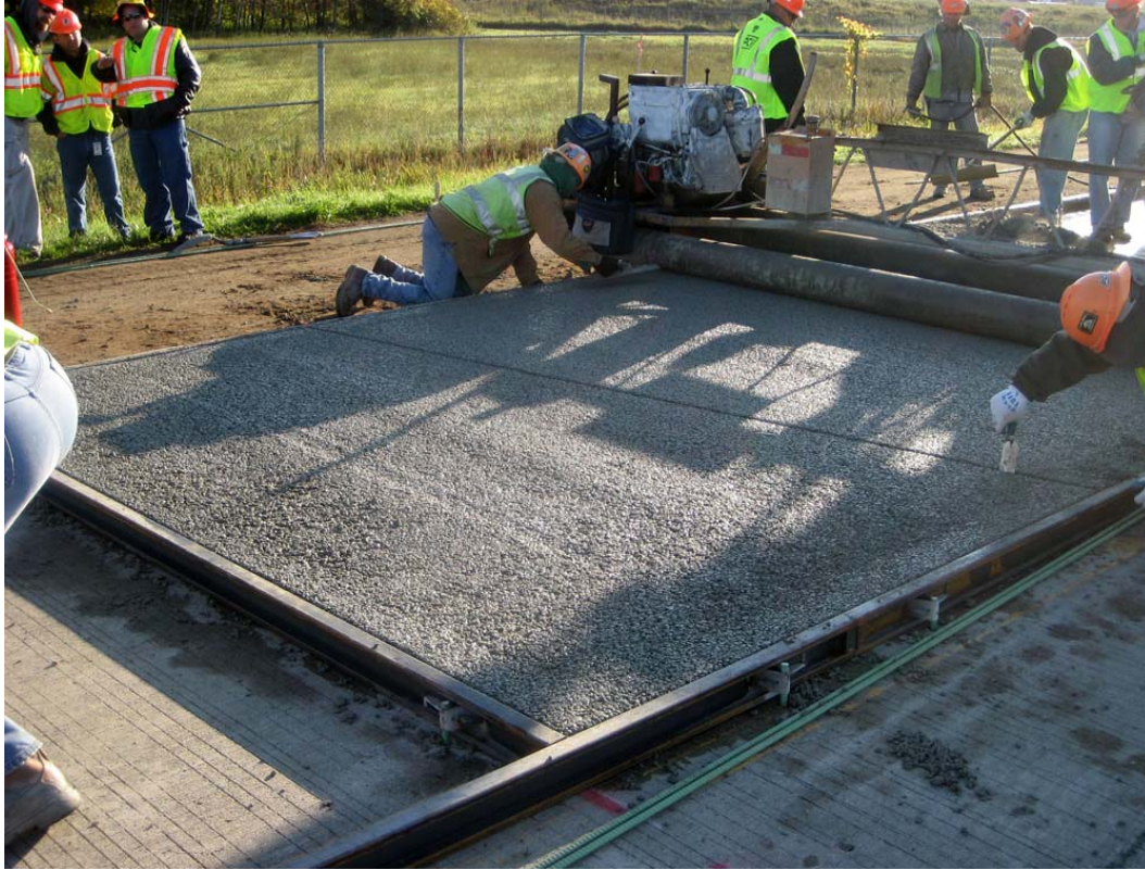
Figure 71. Observation of stretch marking on fresh pavement
