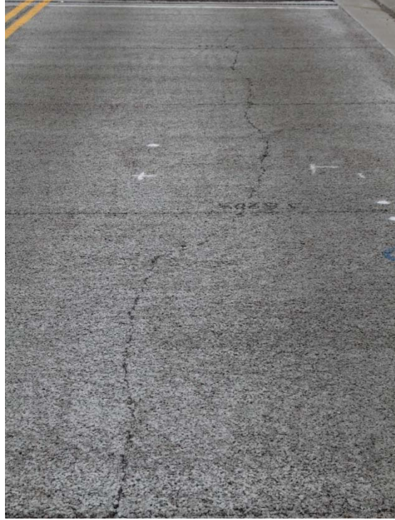
Figure 68. Longitudinal crack from heavy vehicles or loading repetitions
